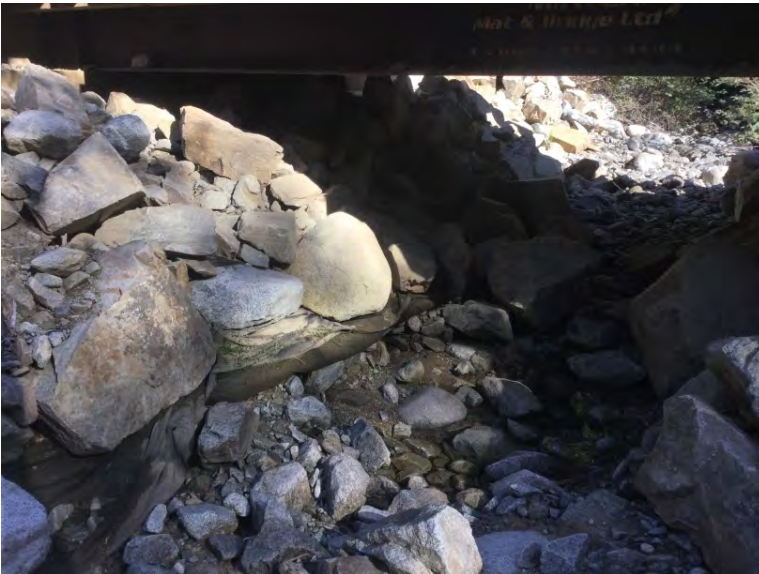
Right bank riprap scour
